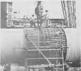
RIGGERS HOOK into the steel-cable lashing wrapped around skid lagging. Five "live" and five "dead" 1½" lines make up the lashing. "Spiders" are constructed in the stack to prevent crushing at this point. RIGGERS TA pass a cable of steel for round of its sostené di roblo. Cinco "live" y cinco "dead" cable di 1-½" in forma e lashing. "Spiders" ta wardé construí den e schoorsteen pa previni machucamento.
